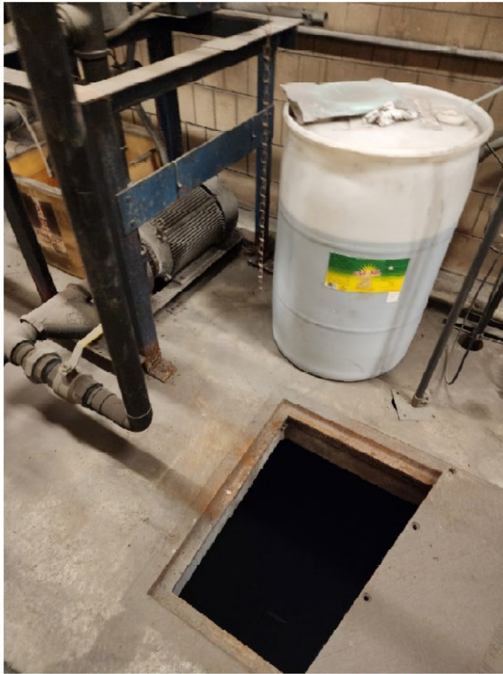
Gray Water Reclamation Tank Manhole 2 of 2
