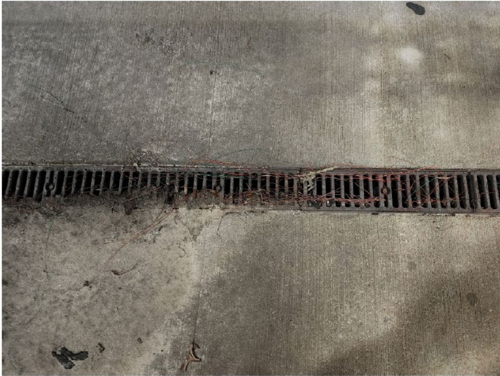
Trench Drain Grate Partially Covered with Debris
