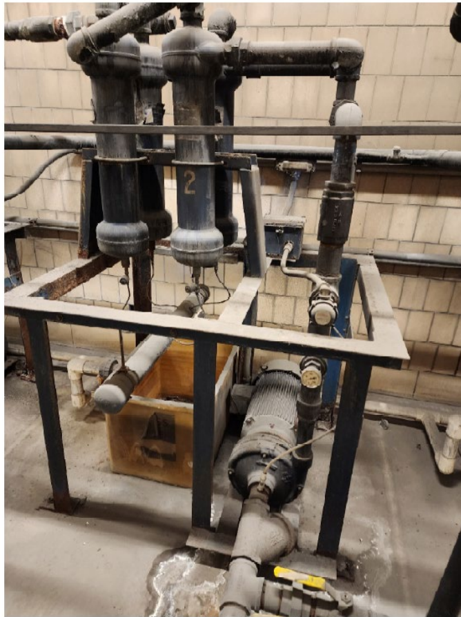
Bus Wash Pump #2
